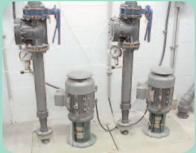
Fybroc Series 5500 Vertical pump installation
