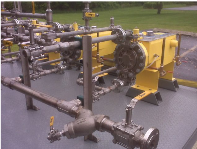
Acetic acid metering pump skid with Milton Roy® Milroyal metering pumps, socket-welded piping, extended valve stems for heat tracing and insulation, and fabricated steel base plate
