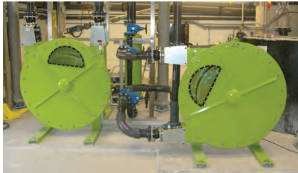
ALH100 handling limewater in a wastewater treatment plant
