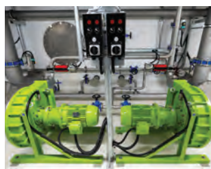
ALH65 wastewater treatment
