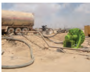
ALH125 crude oil pumping
