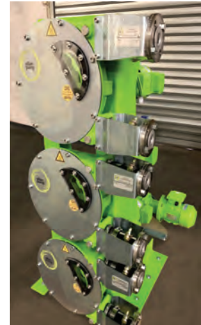
ALH25 pumps stacked, used for the distribution of lime milk in a municipal water treatment plant
